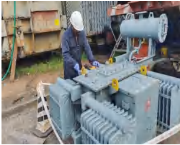
Figure 8: Step down transformer connection to PCB unit
