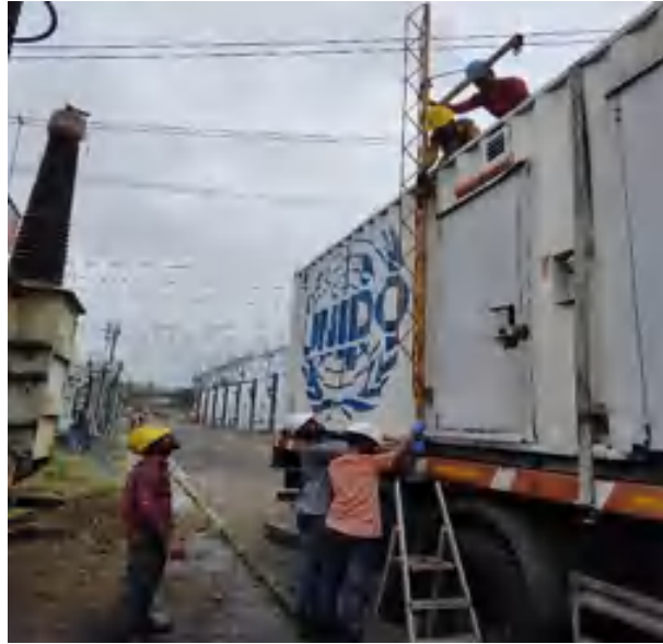
Figure 4: Chain pulley connection to PCB unit
