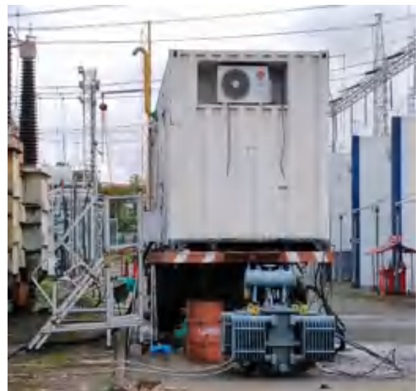
Figure 7: Earthing connections and step down transformer connection
