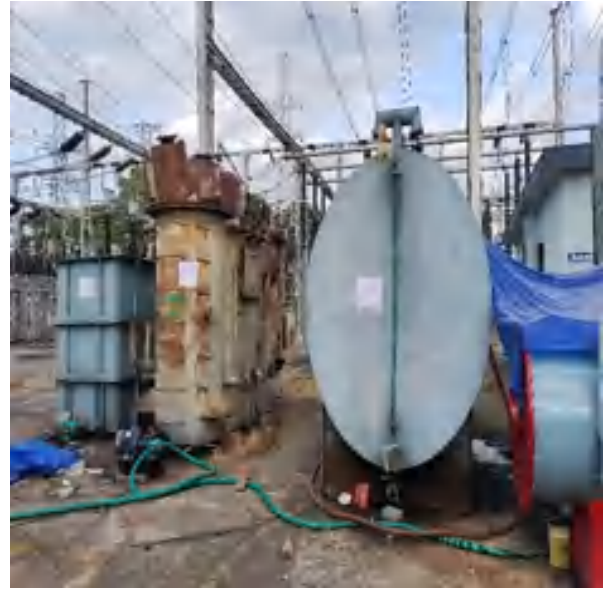
Figure 5: Tank for storage of PCB dechlorinated oil is kept near the PCB unit
