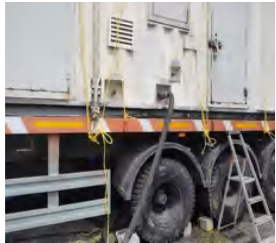
Figure 11: PCB oil loading line connection
