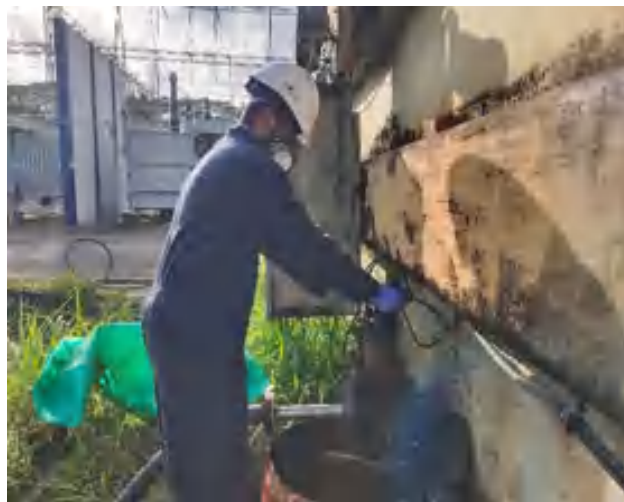
Figure 18: Oil drain connection from PCB contaminated transformer
