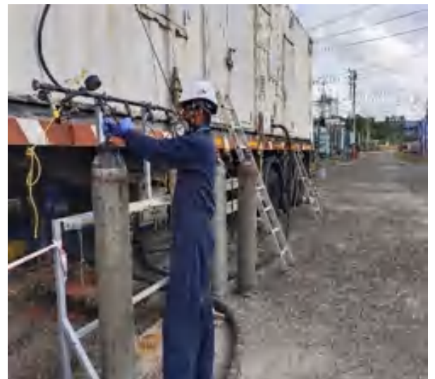
Figure 15: Nitrogen cylinder connection
